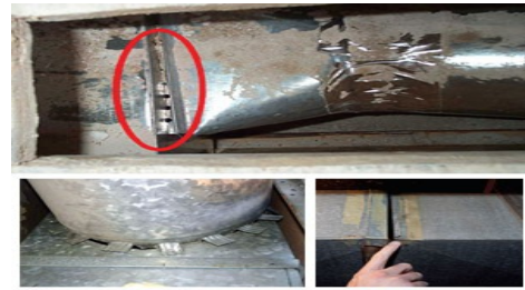
Examples of common duct leaks
