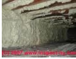
Closed cell foam adhered to foundation wall
