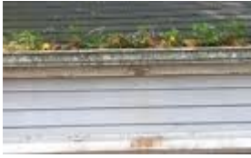
Gutters left unattended add to both roof and wall problems
