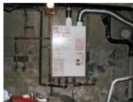
Tankless Water heater
