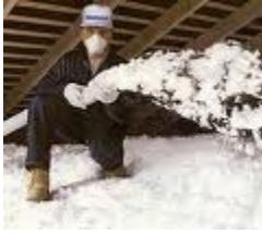
Blown attic insulation will out perform bat insulation
