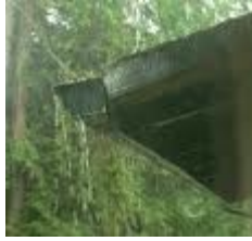
Overflowing gutters dump water directly near your house foundation
