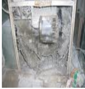
A neglected furnace
